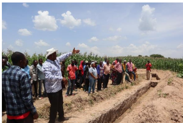
Photo 1: Swai giving a hand-on training to farmers on how to install terraces in the farm. Photo by G.Ndibalema/IITA
