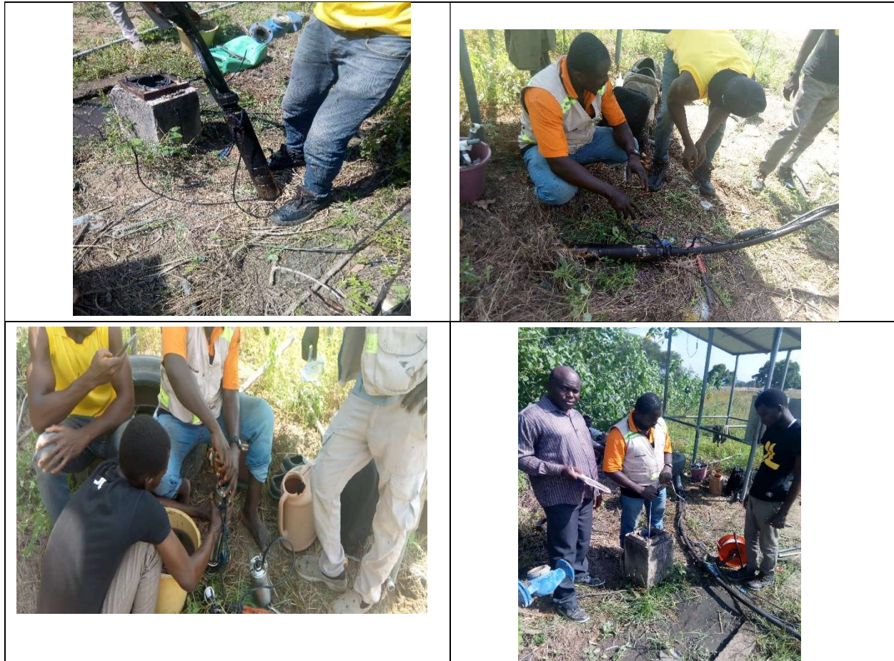
Figure 2: Servicing of the submersible pumps in Gorogo and Sepaat, 2021/2022 season
