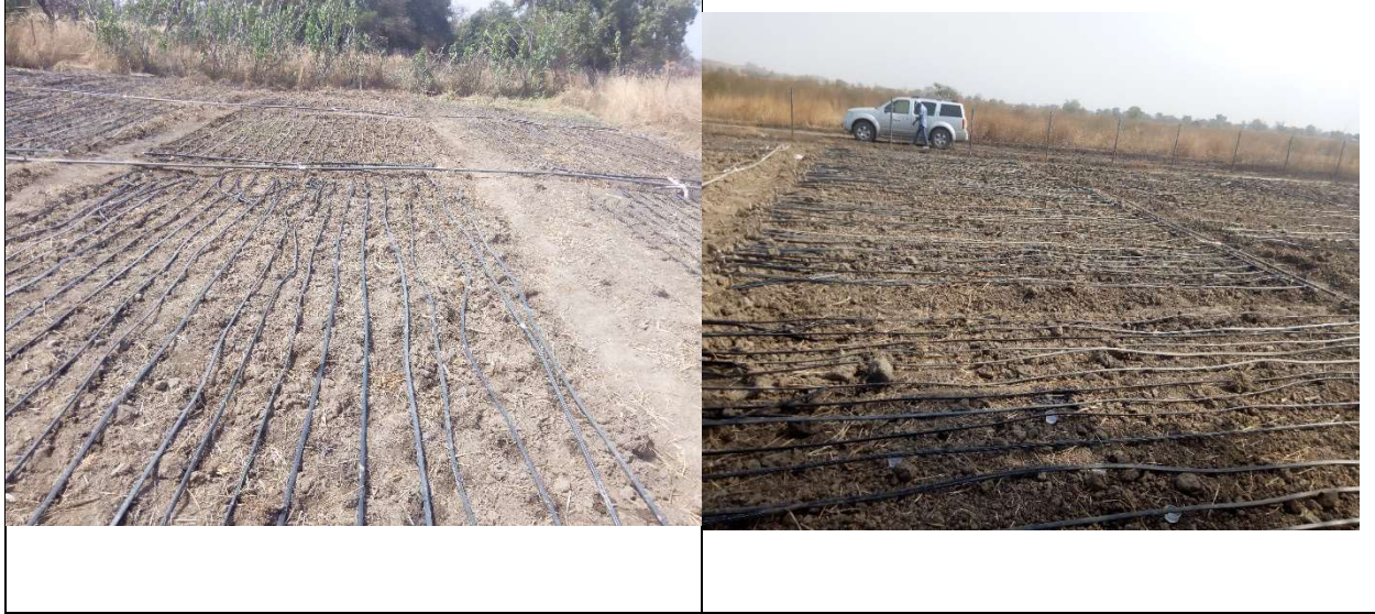
Figure 4: Images of field layout and drip system set up in Gorogo and Sepaat experimental fields, 2021/2022 Season
