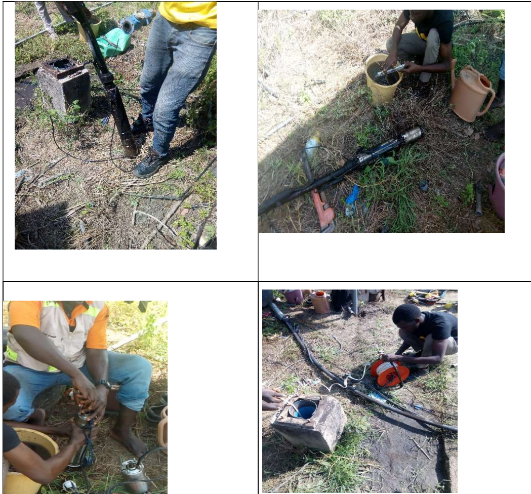
Figure 6: Servicing the submersible solar-based pump (Picture by H.E. Igbadun)
