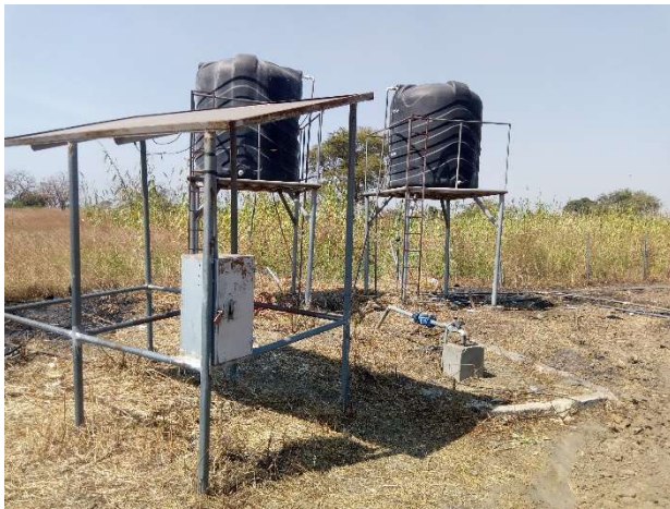
Soil Panel with Overhead tanks (Picture by H.E. Igbadun)
