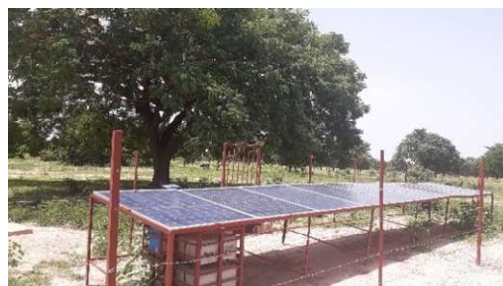
Picture 1b. Solar panels in the technology park in N'Golonianasso.
