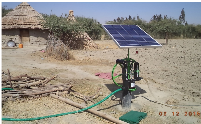
Picture 1: Piloted solar water pumps.
